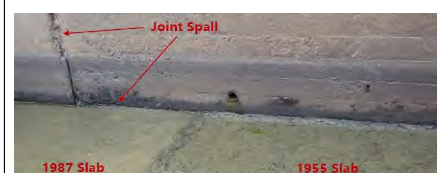
Concrete deterioration on downstream vertical edge of weir on 1955 basin slab. Oct 23, 2019
