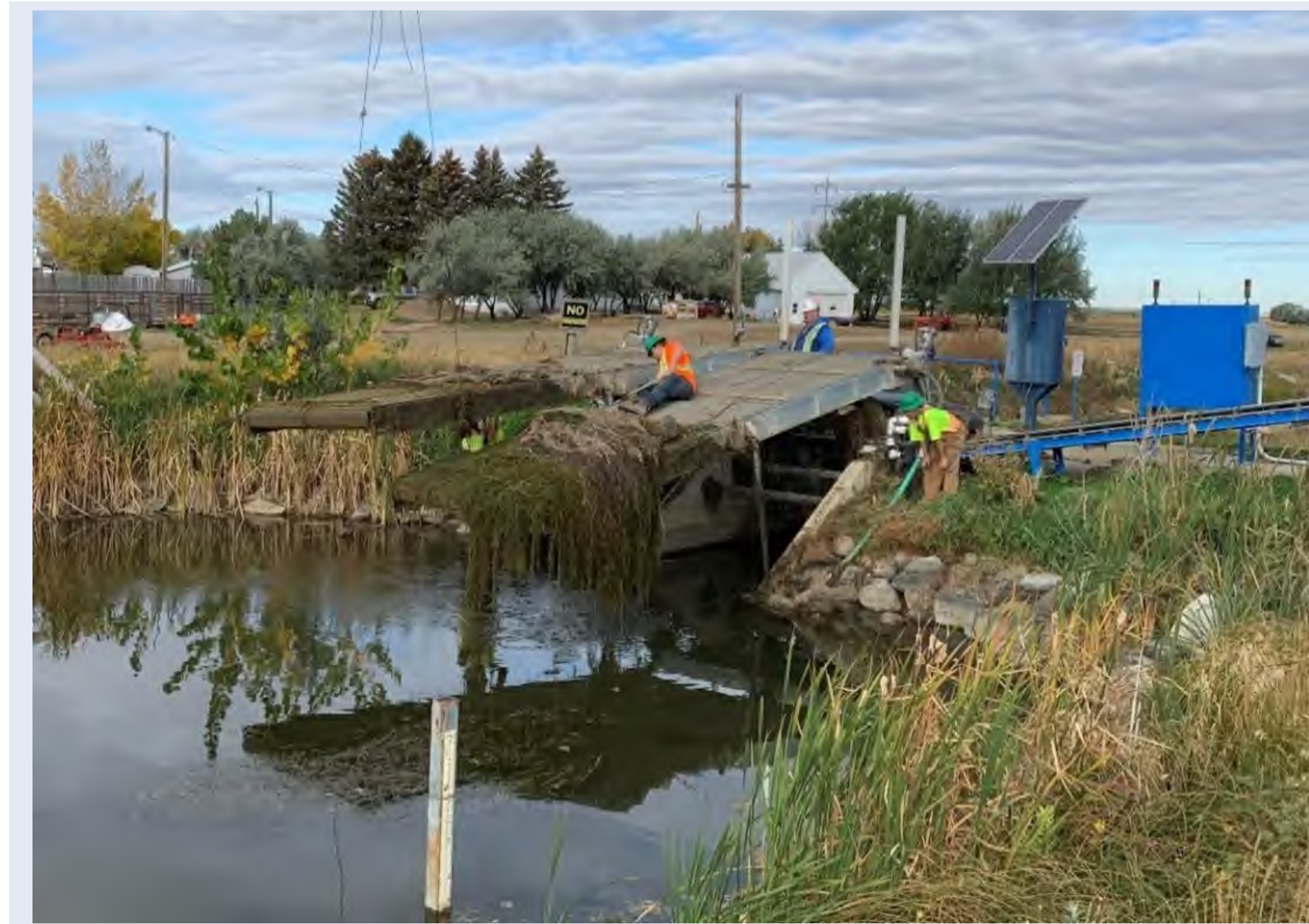
Big Bend Main Canal Inlet Structure Prior to Replacement (Start of Horsefly Spillway – Phase 1)
