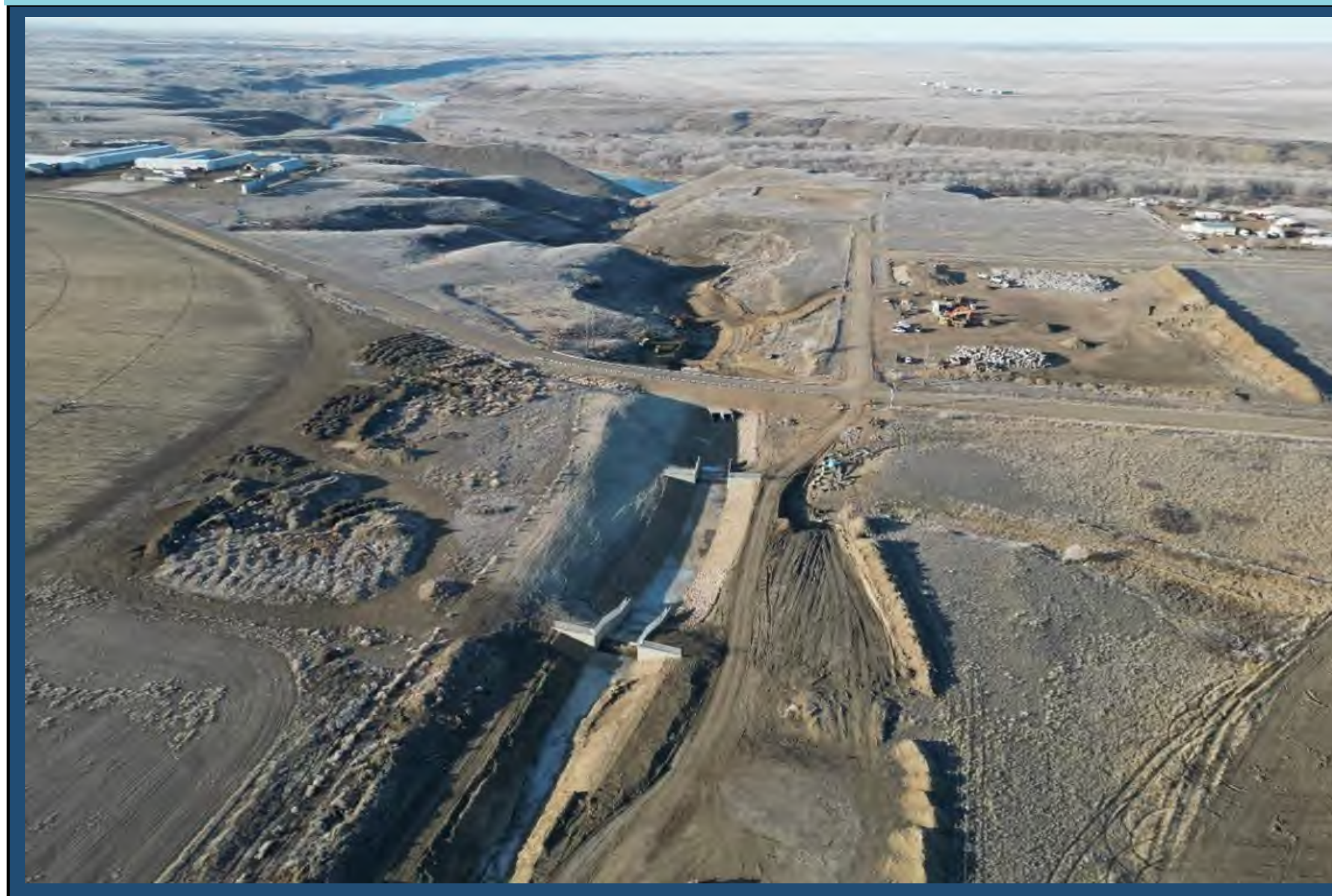
Construction Underway in the Drain Channel and Down the Coulee to the Oldman River (MPE, a Division of Englobe)
