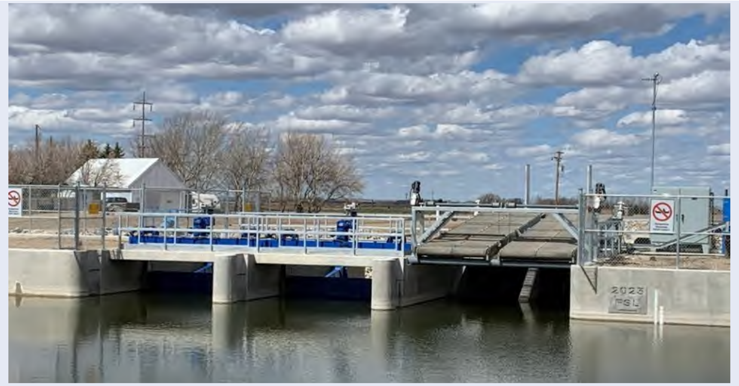
Big Bend Main Canal Inlet Structure After Replacement in May 2023 (Horsefly Spillway – Phase 1)
