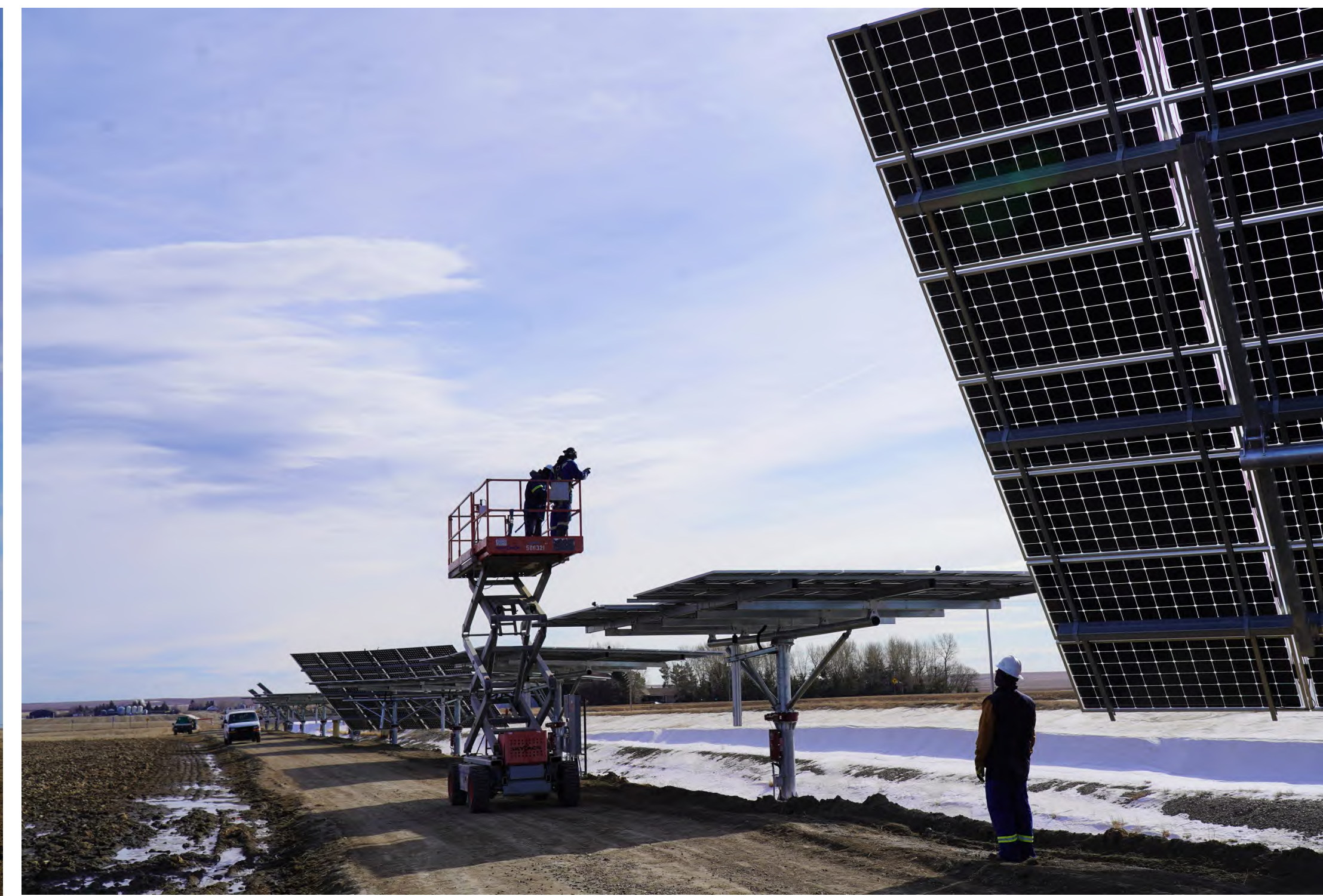
Bow Island Lateral 12: The 705.6 kW (DC) system consists of 400 Watt solar modules with real time monitoring. The system allows SMRID to supplement its electricity with solar electricity generated on-site.
