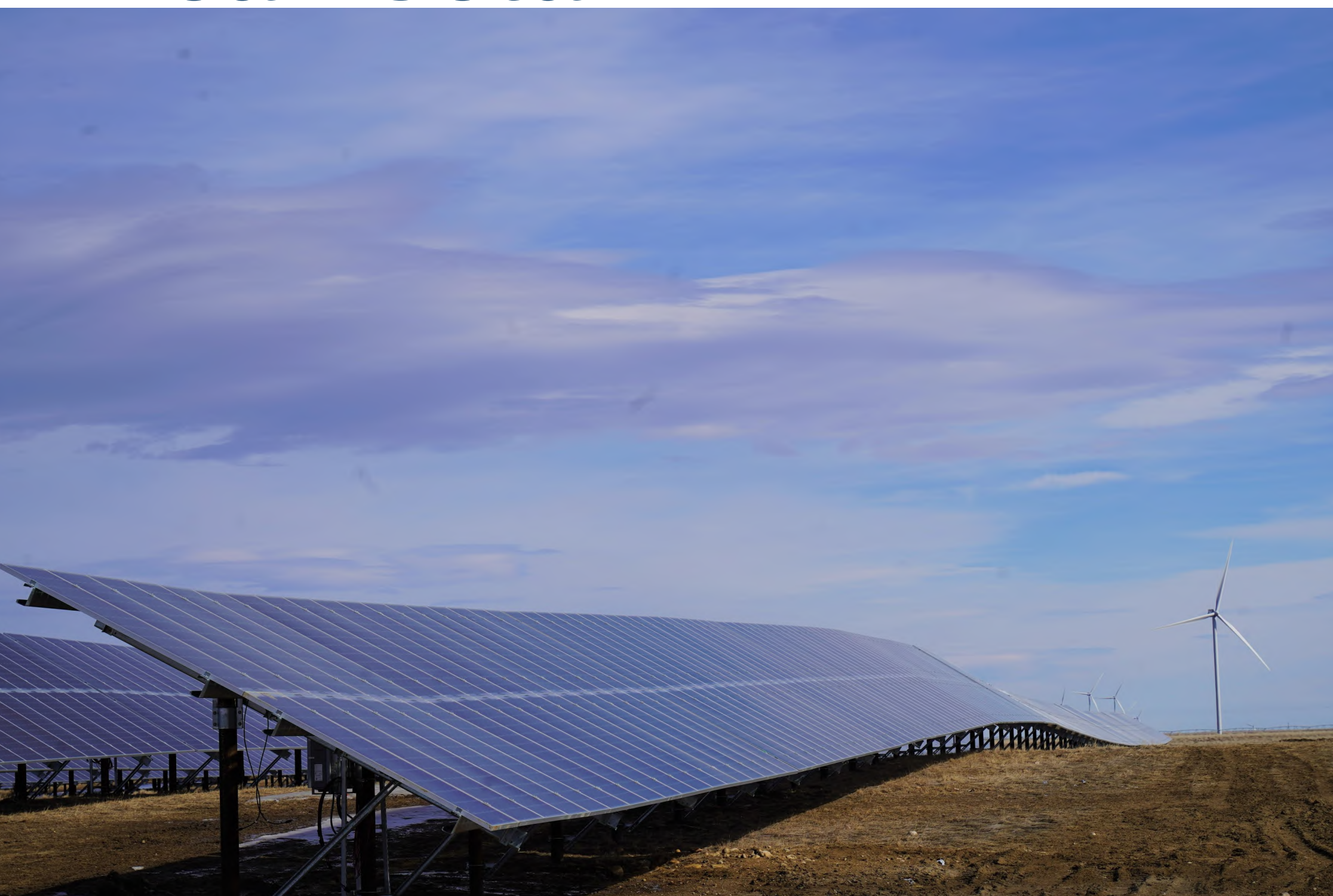
40 Mile: The 1747.20 kW (DC) system consists of 400 Watt solar modules with PV power optimizers and real time monitoring
