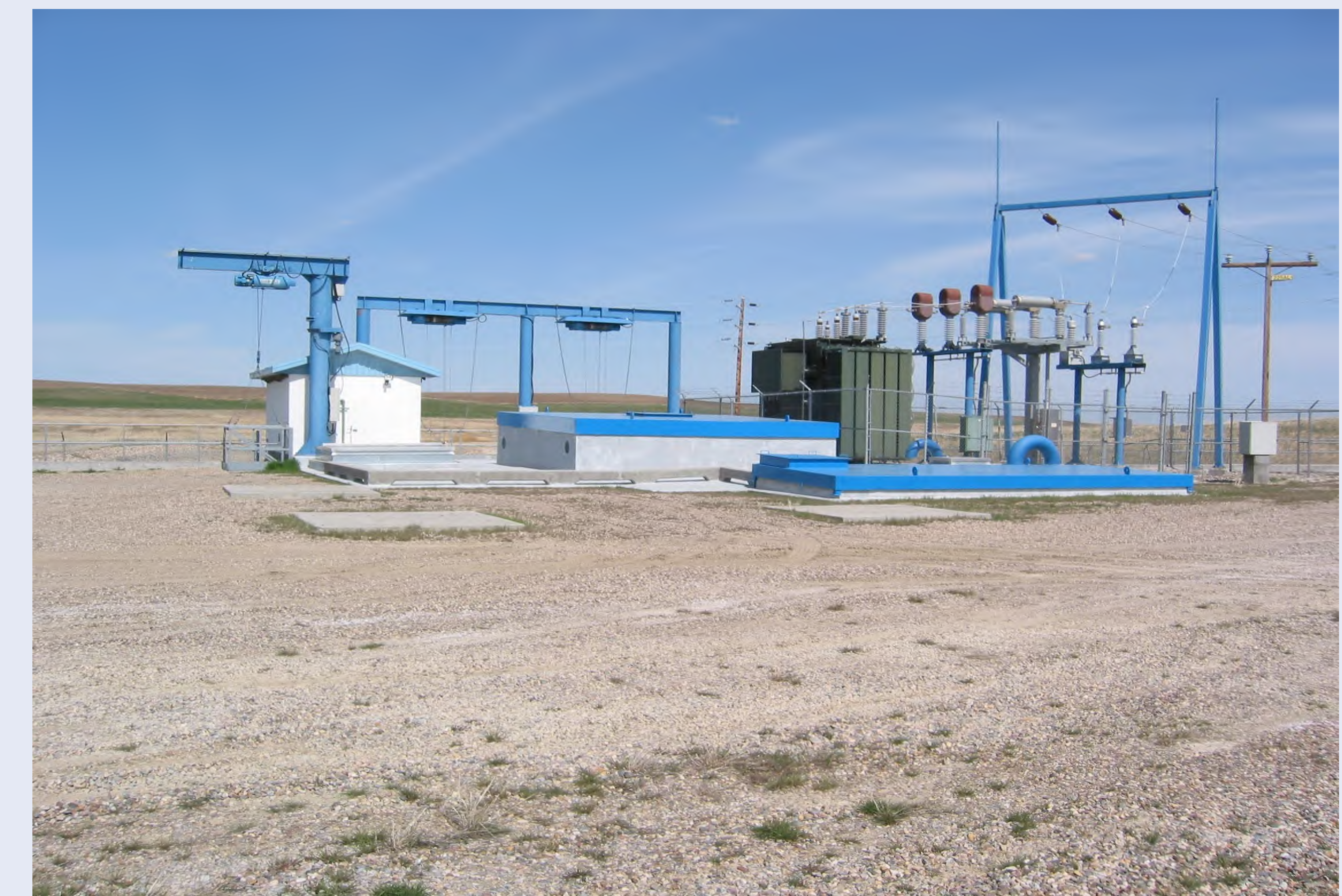
Raymond Hydro is our largest Hydro facility at 18 MW and has a vertical Kaplan turbine and a head of 43.9 m
